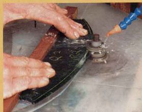
The stoneworker’s turn. Anderson mounted each template on a rough-cut stone blank and used a bearing-guided diamond bit in a router-table setup to create the bead. A jet of water kept the cutter cool.
